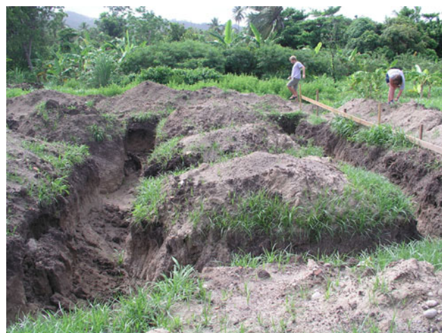
Fig. 5 Series of trenches dug by locals into the Pearls site in Grenada to apparently build a residence. It is clear, however, that this also provided an opportunity for others to collect artefacts (June 2005)
